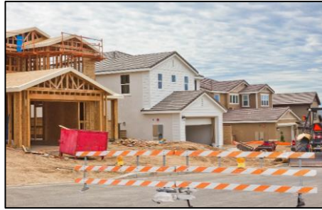
Streets In – streets appear to be poured for the entire section, but are not accessible to verify
